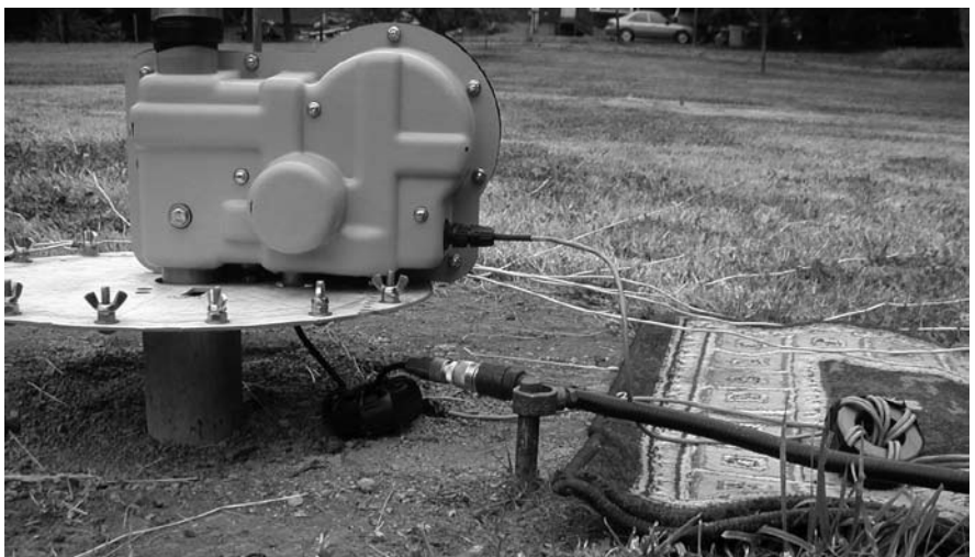
Figure 4A — Chokes installed in the feed line and control cables at the base of the antenna.
